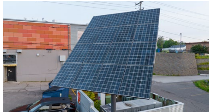
16-panel solar array at the Hillside store.
